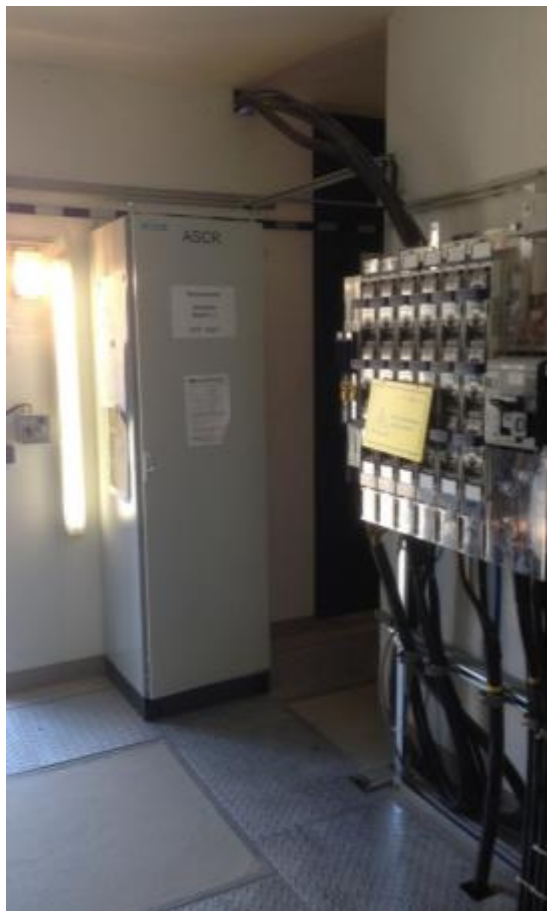
ICT-Schrank in Transformatorstation
