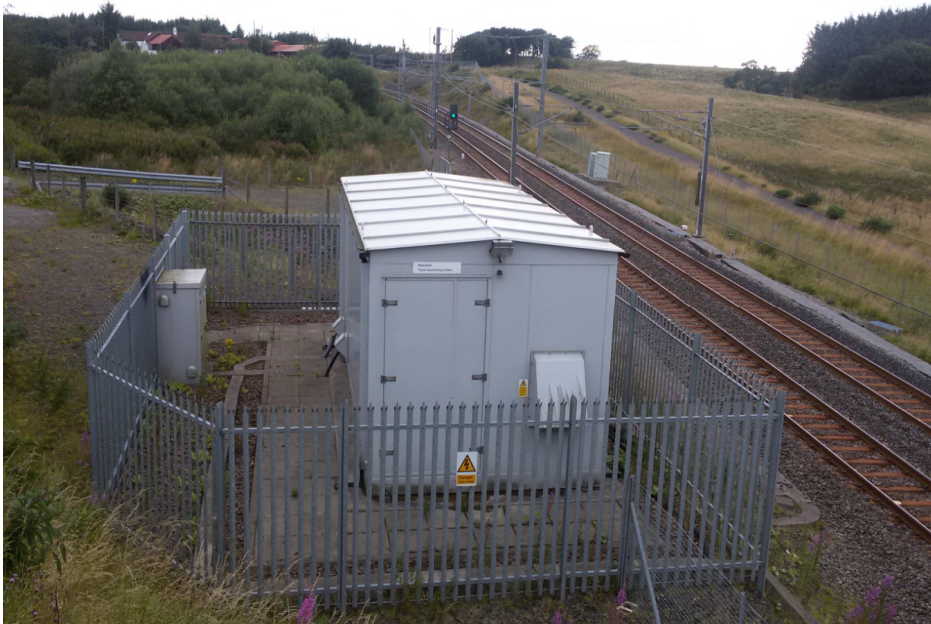
Track Sectioning Cabin, Raiziehill Schottland
